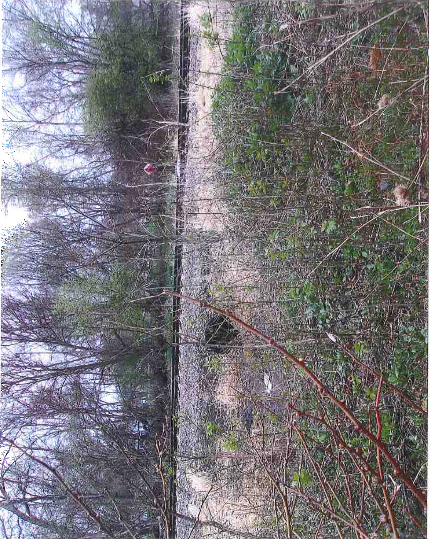
LOOKING DOWNSTREAM @ RR MAINLINE, SURFACE TUBE DRAINS INTO DD86 TILE
